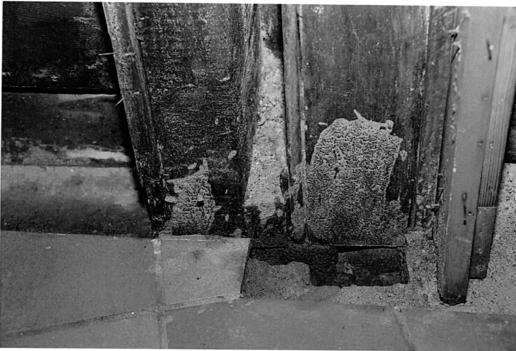
Photo 8 of 14: Basement, south wall beaded post with later infill and stone sill. 9/8/2016
